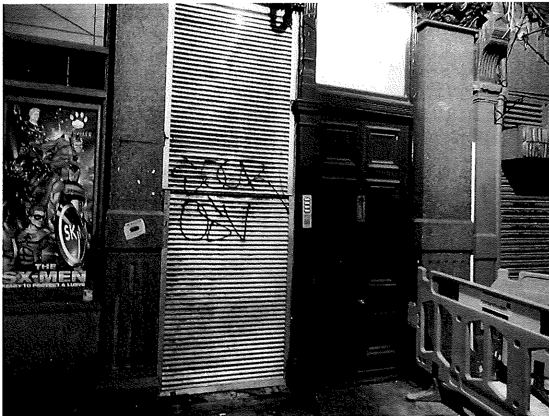
Figure 3: Mechanical plant louvres in Tisbury Court. The plant was operating thought the night.
